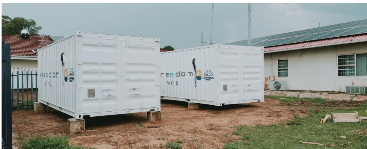
Westlake City Power offices (538kwp, 1MWh battery)
